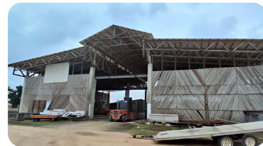
In Zanzibar, construction developer (and Biobased Construction East Africa Coalition member) CPS has built a manufacturing facility to process local timber with local labour for its Fumba Town development.
